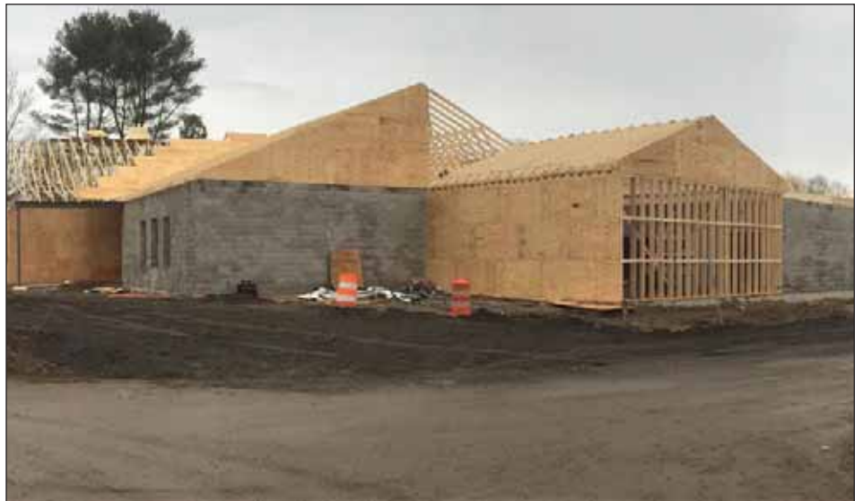
The new police station building at 64 Middle Road in Acushnet is taking shape in this photo from December 22. From the Acushnet Police Department Facebook page.
